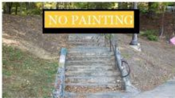
The steps and handrails from Campus Drive to Pettigrew Street (see above)
